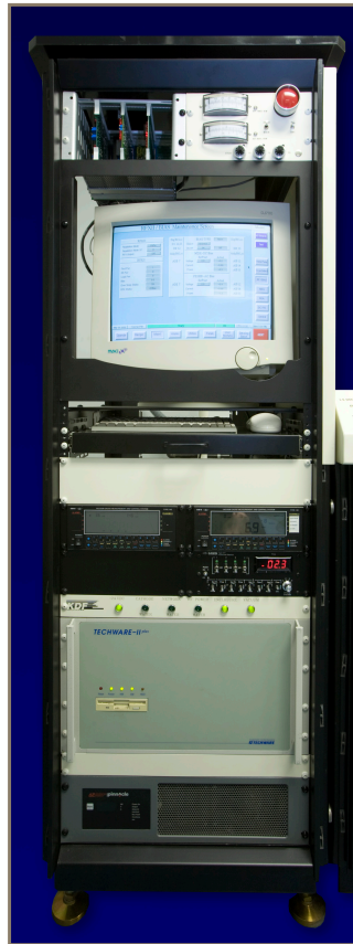
Old GT controller tower
