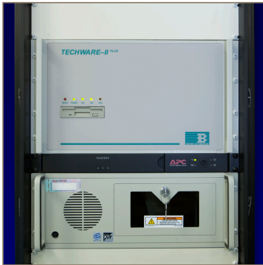
Old NT Techware controller tower
